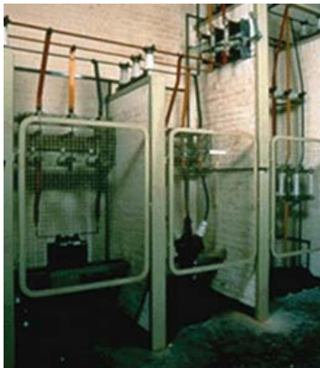
Fig.1: open cells in substation
